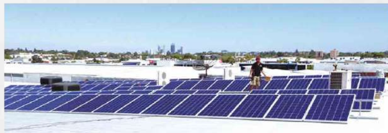
15kw Perth, Australia 📍
