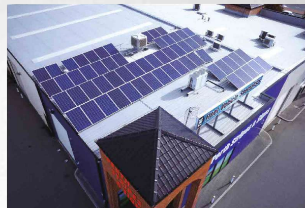
15kw Perth, Australia 📍
